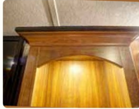
07. ELEGANT CROWN MOLDING ABOVE THE KITCHEN & BEDROOM CABINETS
