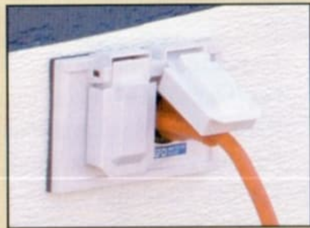
Exterior 110 Volt Receptacle. G.F.C.I. Protected
