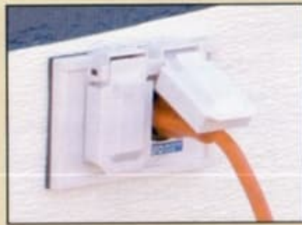
Exterior 110 Volt Receptacle. G.F.C.I. Protected
