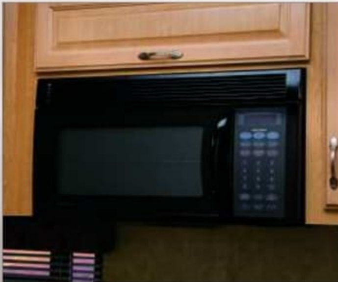
▲ A 30-INCH, RESIDENTIAL-STYLE MICROWAVE IS MOUNTED ABOVE THE STOVE FOR ADDED KITCHEN CONVENIENCE AND EFFICIENCY.
