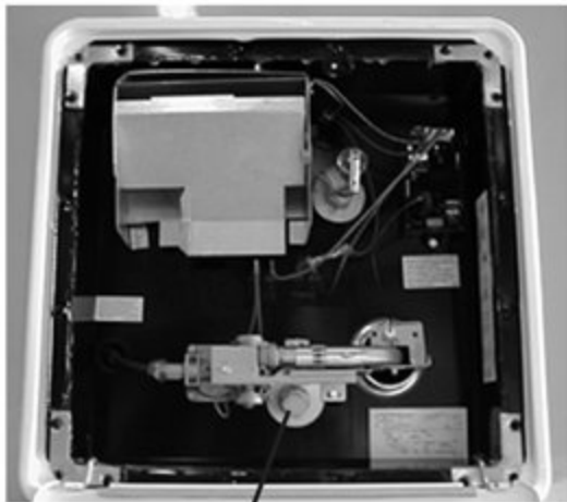
Water Heater Drain Plug
