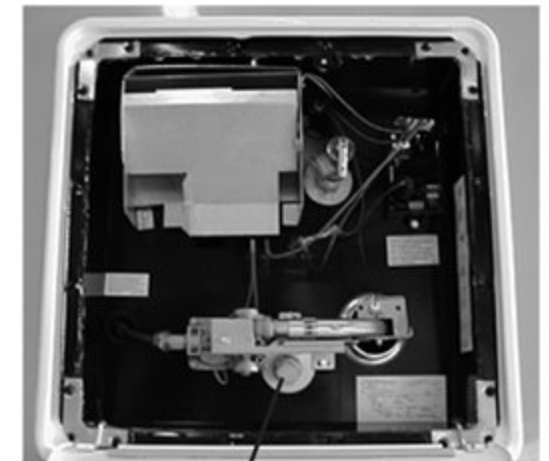
Water Heater Drain Plug
