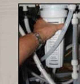
The city water fill is filtered. Cartridges can be changed through an access hatch
