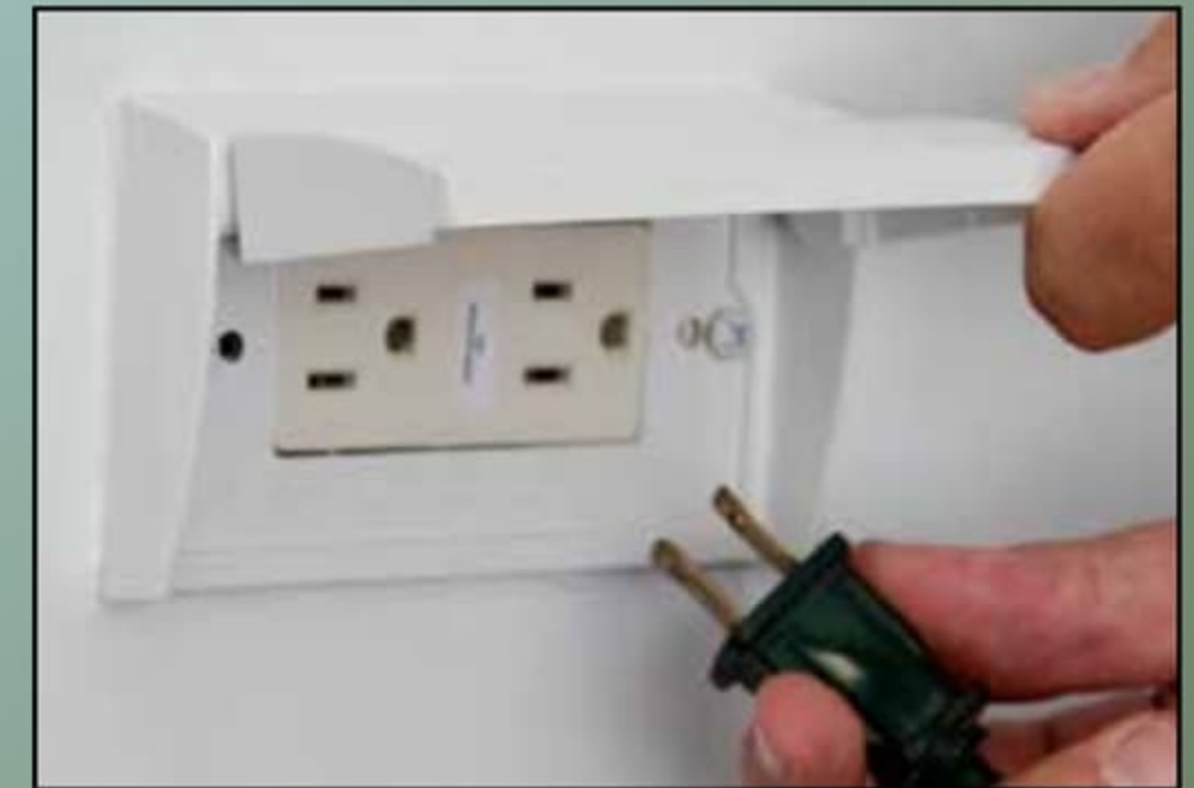
Convenient Outside GFCI Protected and Covered Outlet.
