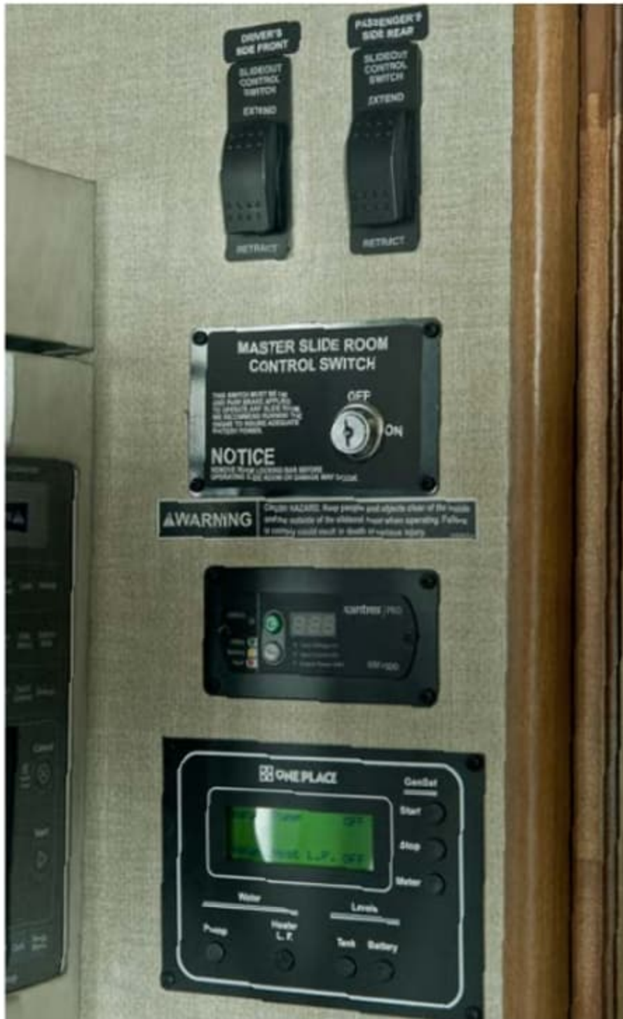
The OnePlace® Systems Center lets you monitor and control key systems from one convenient location.
