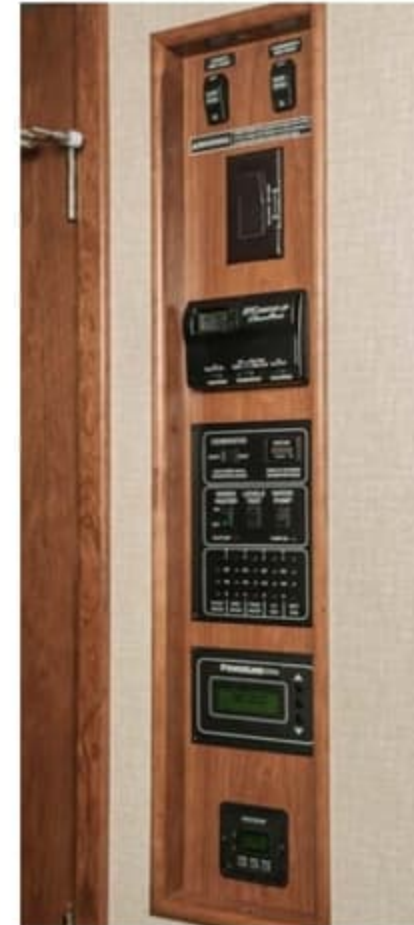
Important gauges, switches and controls are all centrally located in the OnePlace® Systems Center .
