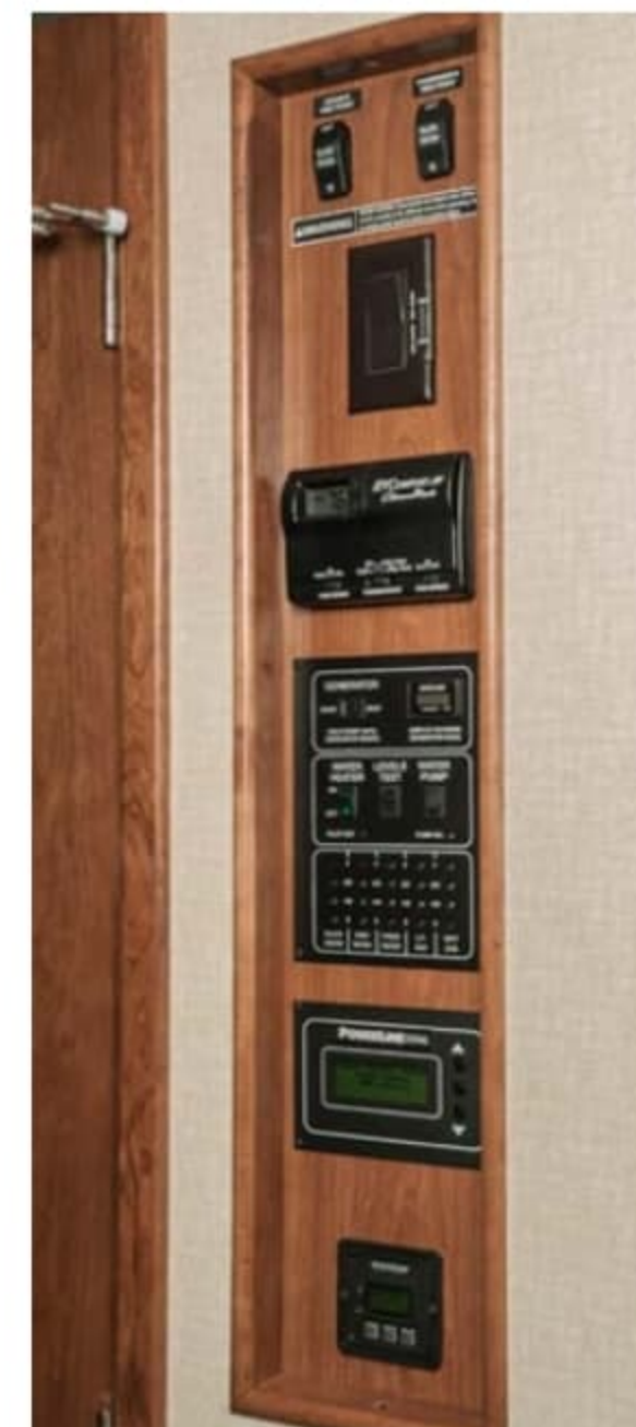
Important gauges, switches and controls are all centrally located in the OnePlace® Systems Center .
