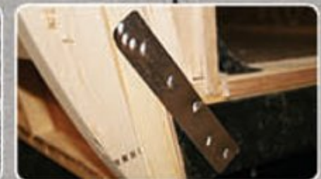
HURRICANE STRAP REINFORCED ROOF & WALLS
