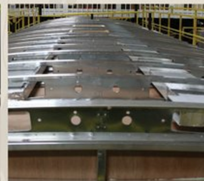
Walkable steel truss roof system
