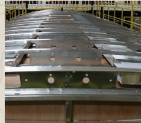
Walkable steel truss roof system
