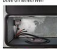
Generator Prep (Standard 27KB, 29SS)
