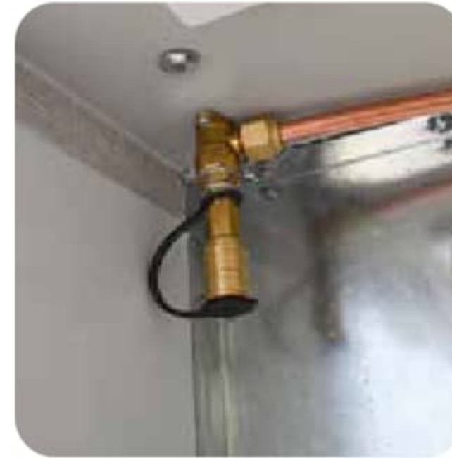
Exterior Propane Connection
